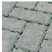
Permeable keyblock paving
