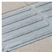
Tactile corduroy paving
