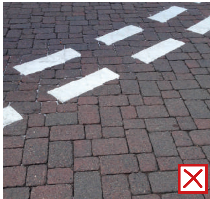
No white lining to block paving.
