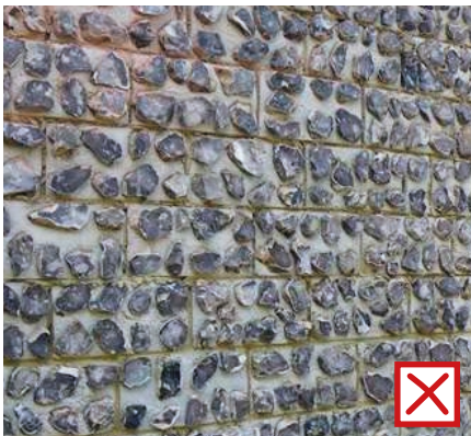
Flint panels to walls will not be acceptable.
