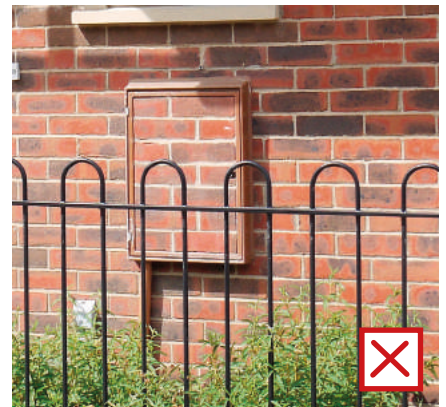
Poorly masked gas meter boxes are not acceptable
